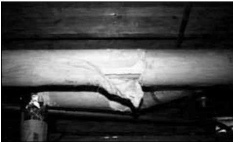
Minor Damage to Pipe Wrap
